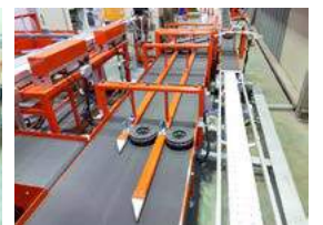
Empty Tray Returning Standby Conveyor
